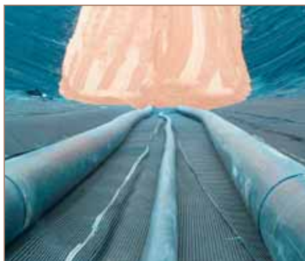
Leachate Collection System pipes sitting on top of panels of Uniaxial Geogrid at the West Side of the Cell.
