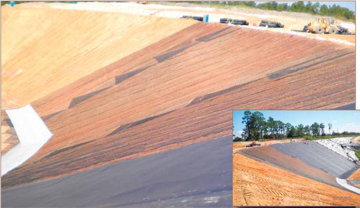
First panels of Biaxial Geogrid, GCL, and Geomembrane deployed at the East Side of the Citrus County Central Landfill Cell 3 Expansion Project.
