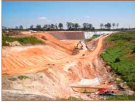
It took 3 months of stripping, excavating, and grading on the Cell before geosynthetics were ready for deployment.
